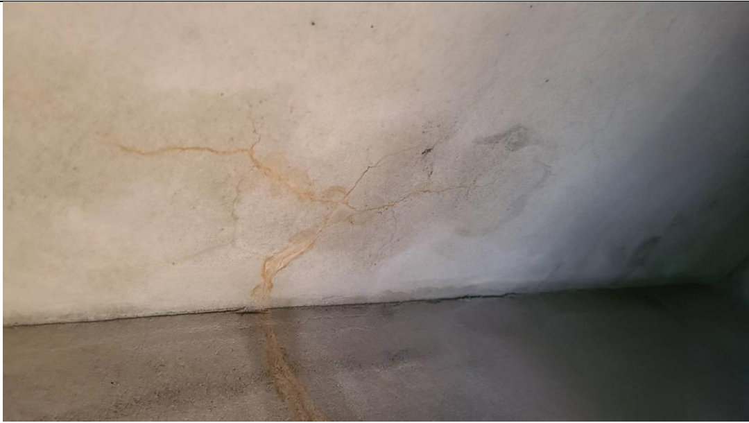
19（施工前）赤崁所待勤室大門上方漏水照片
