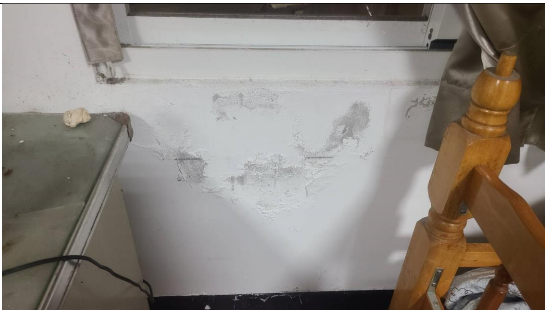
17 (施工前)赤崁所窗框壁癌照片
