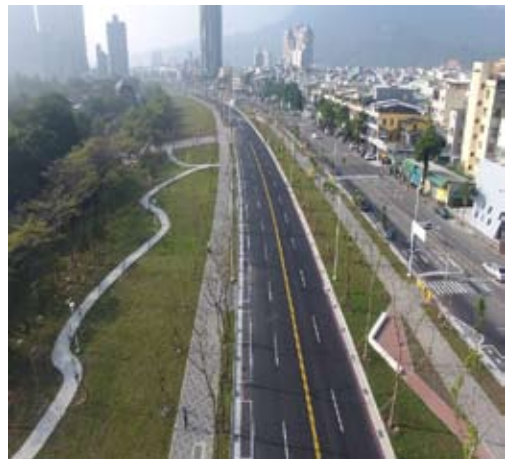
Kaohsiung City Railway Underground Project station park lane engineering – Mingcheng 4th Road to Museum of Fine Arts section
