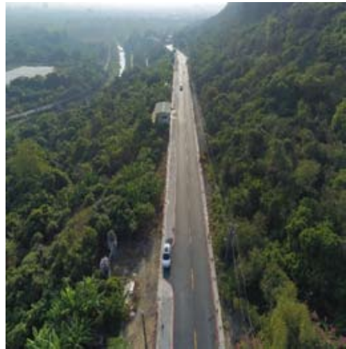
Gangshan District Access Road for Kaohsiung Highway No.28 and No.29 (Shuiku Road and Dazhuang Road) Widening and Improvement Project (Tender A)
