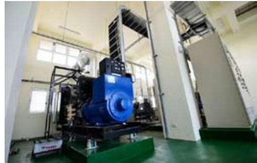
Pumping station on Jhongjheng Road in Zihguan
