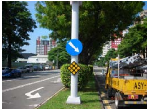
Added Regulatory No. 18 and Warning No. 3 signs
