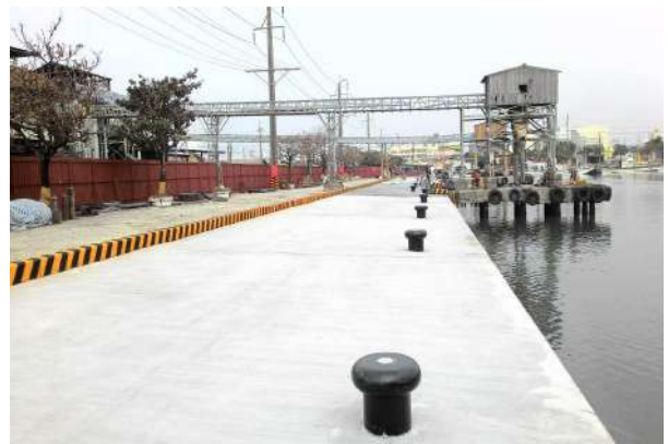
Basic improvement project for facilities at wharves in coastal and offshore areas in Singda Harbor
