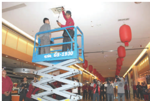
Inspect fire-safety equipment.
