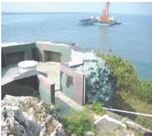
Landscape improvement works at the military sentry box near the Syongjhen North Gate and the surroundings thereon – Before
