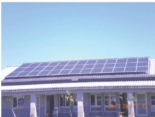
Current status of the solar photovoltaic systems installed in Daai Park in Shanlin District
