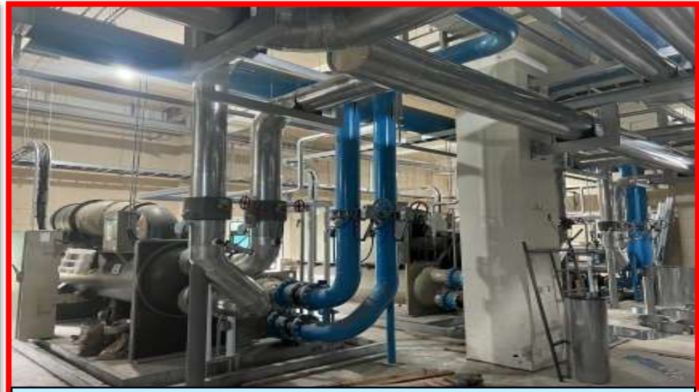
5°C 冰水主機群(CH-1/2/3*2+1台)
