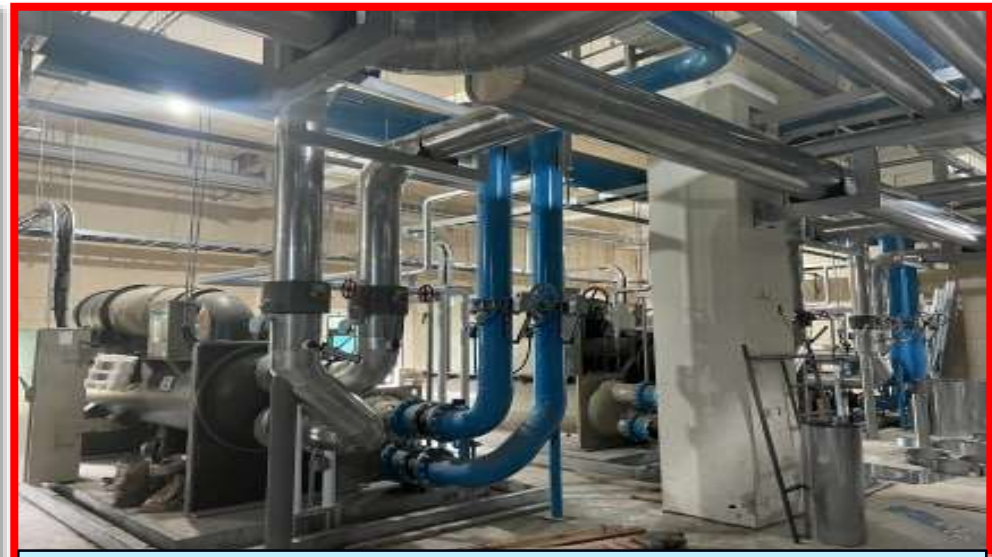
5°C 冰水主機群(CH-1/2/3*2+1台)
