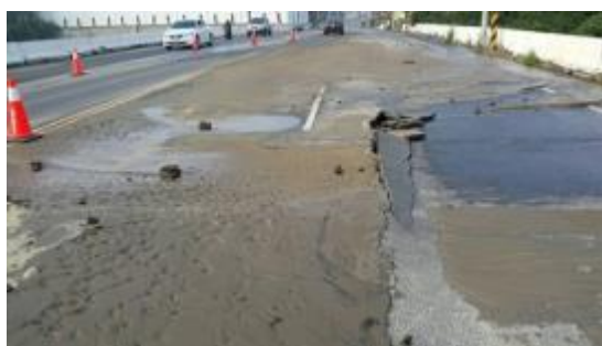
(a)開運橋頭(永康側)破管
